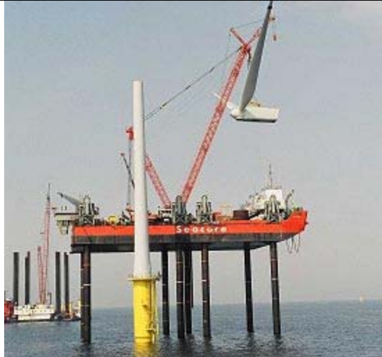
Figure 1 – Installation of a wind turbine at North Hoyle off the coast of North Wales.
